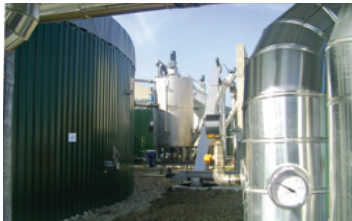
Bondeno is the site of Italy's largest bioenergy park for the production of biogas.
