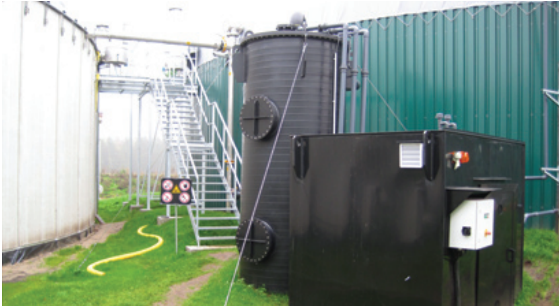
Biogas plant operators achieve high purification with the new external desulphurisation plant.
