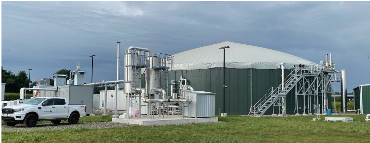
Oakridge Dairy Biogas Plant, Online (Gas to Grid): 9/14/2023
