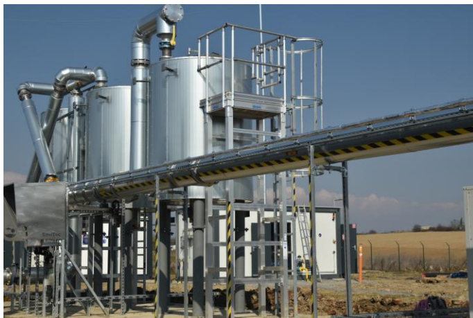
Thanks to this plant, 750 Nm 3 /h of biogas is upgraded to biomethane. In future, up to 1,300 Nm 3 /h is set to be processed. (Photo: EnviTec Biogas AG)
