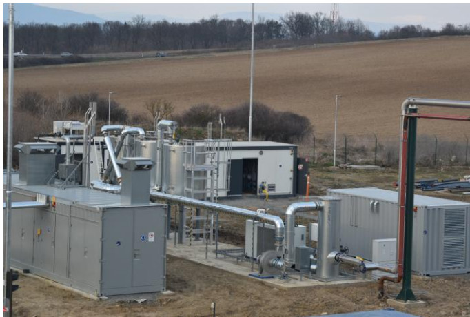
The EnviThan gas upgrading plant with a capacity of 417 Nm 3 /h is EnviTec Biogas’s second biomethane project in Slovakia. (Photo: EnviTec Biogas AG)
