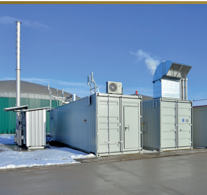
← State-of-the-art hollow fibre membranes are used in EnviThan gas upgrading plants.
